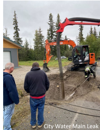
City Water Main Leak
